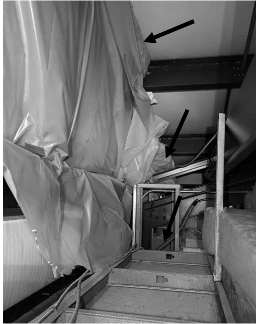
Figure 1. Example of breaks in the air barrier of the shell of the building.
